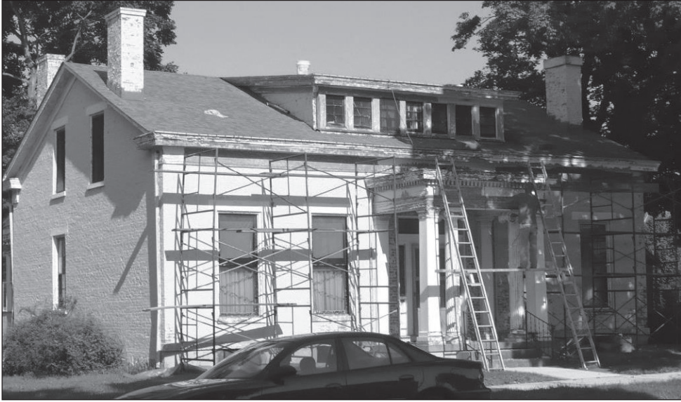
The house at 912 Main Street in 2009 getting ready for major renovation and restoration work inside and out. The old gray paint was removed with a chemical peel so as to not damage the bricks.
