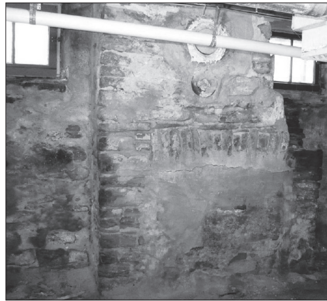
The bricked up hearth in the basement was an unexpected and curious find.
