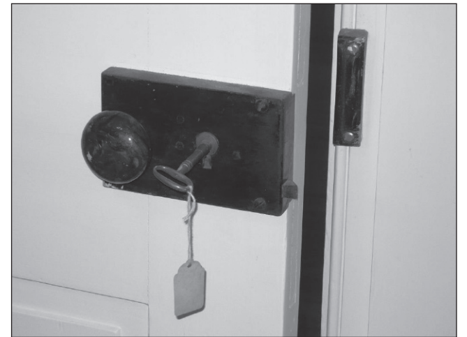
Throughout the house the doors still retain their original hardware and locks.
