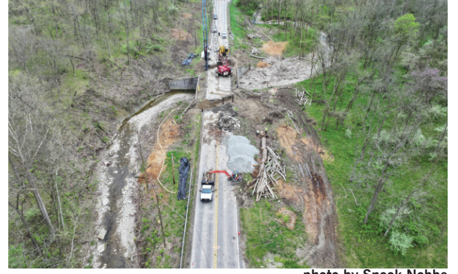
A view of the bridge work being done on St. Rd. 1. photo by Snook Nobbe
